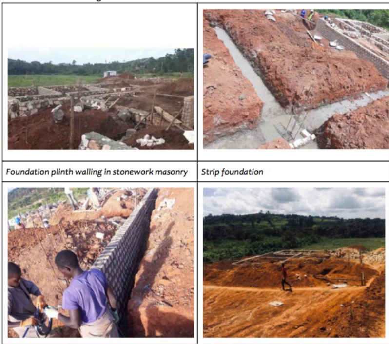
excerpts from the construction of the girls domitory project that is on going
